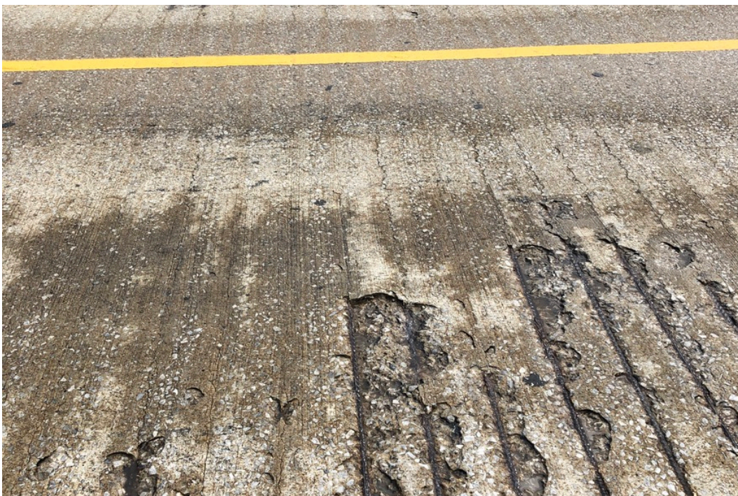
Deteriorated concrete deck Ski Cove Bridge
